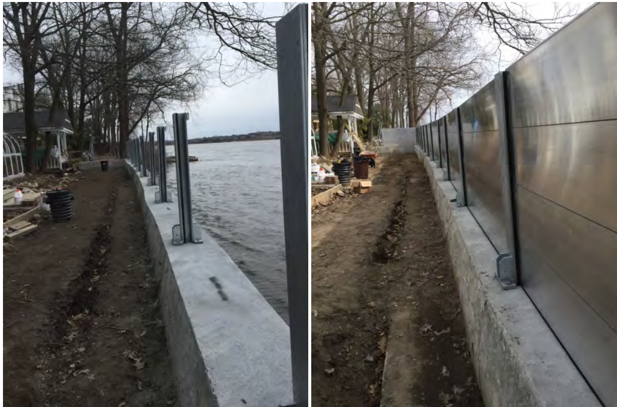
Photograph 5-2: Demountable Flood Wall Foundation (Left) and Erected Barriers (Right) along the Ottawa River (photo from Flood Control Canada)
